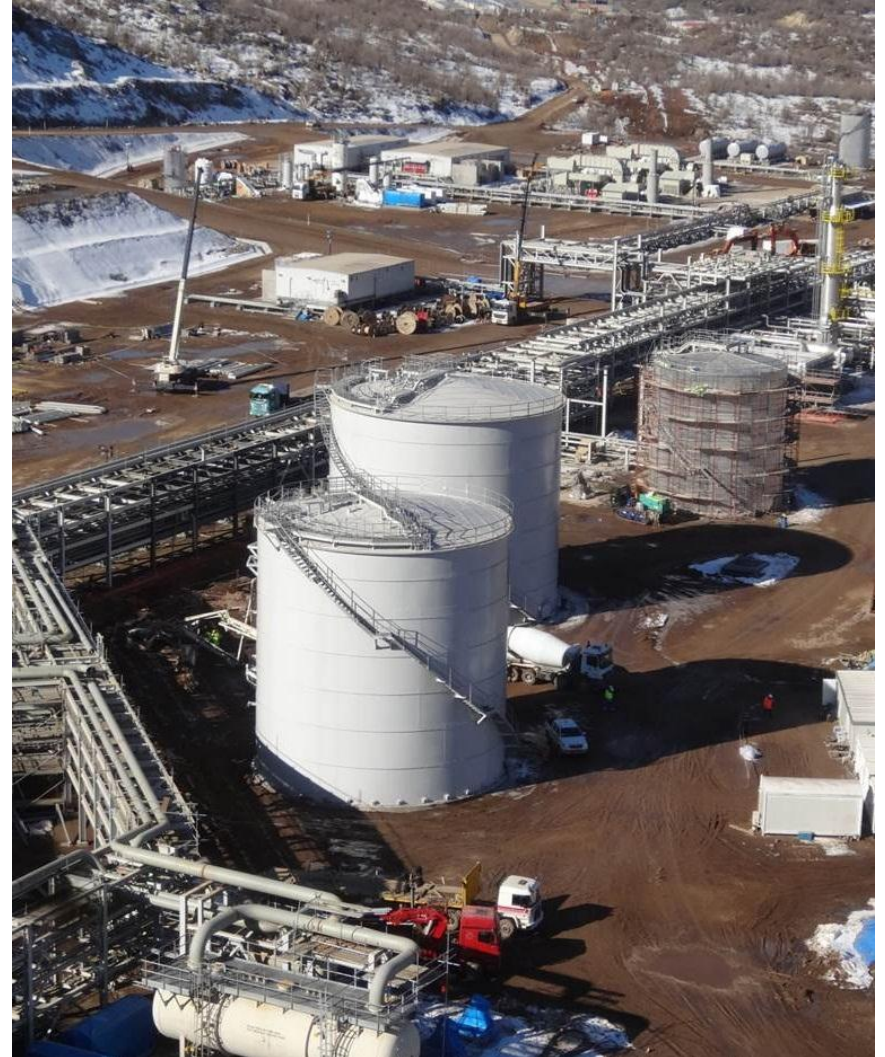
Progress at the 30,000 barrel per day Phase 1 production facility
